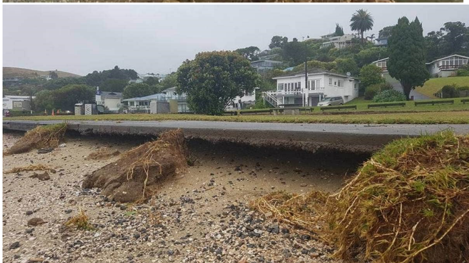
Figure 18: Photos of 2018 storm event road erosion Maraetai Coastal Road (Source: unknown)
