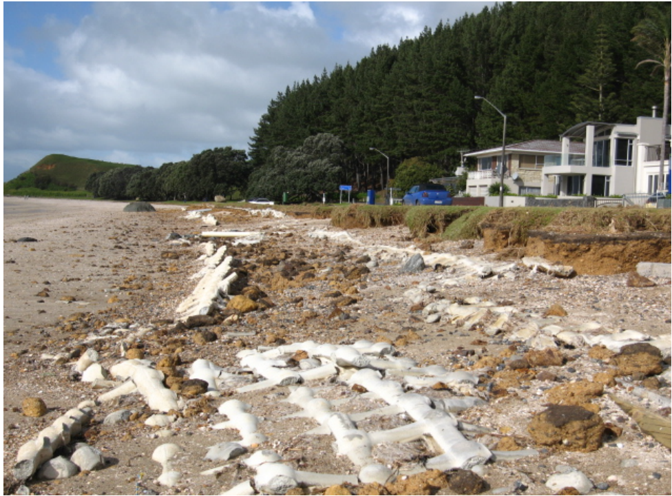
Figure 15: Failed revetment wall at Maratai Beach (Source: Auckland Regional Council)
