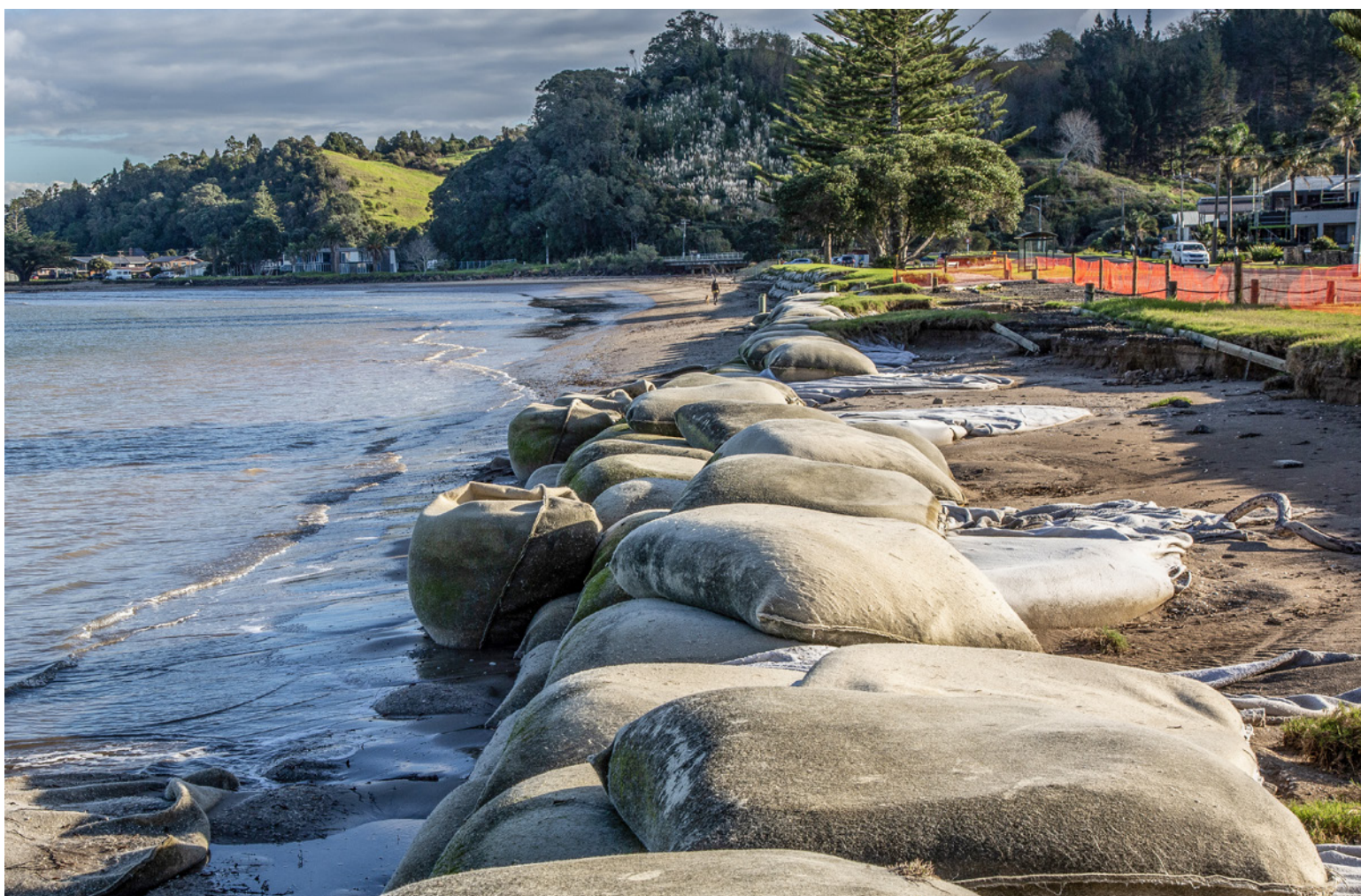
Coastal erosion at Buffalo Beach, Whitianga
